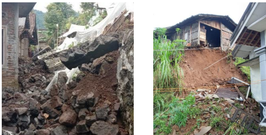
Figure 6. Documentation of Landslide on Built-Up Area in Banyubiru Sub-District
