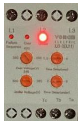
Gambar 11 Phase Failure Relay terhadap tegangan Under
