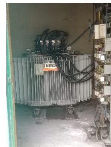
Gambar 2. Transformator Gardu KSBI
