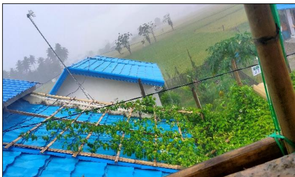
Figure 7. Vegetation Roof Cover Condition in January
