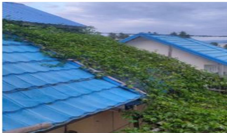
Figure 11. Vegetation Roof Cover Condition in March
