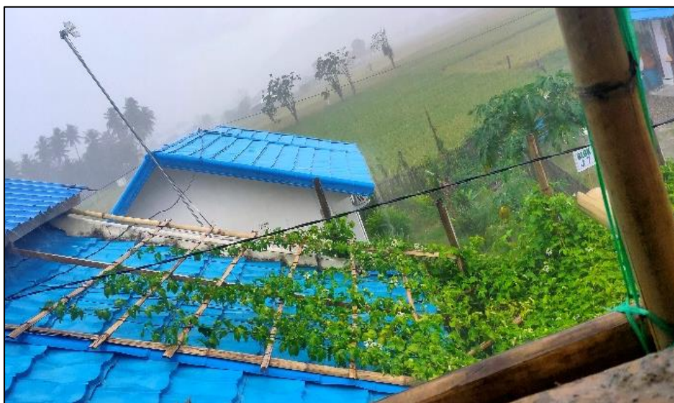
Figure 7. Vegetation Roof Cover Condition in January
